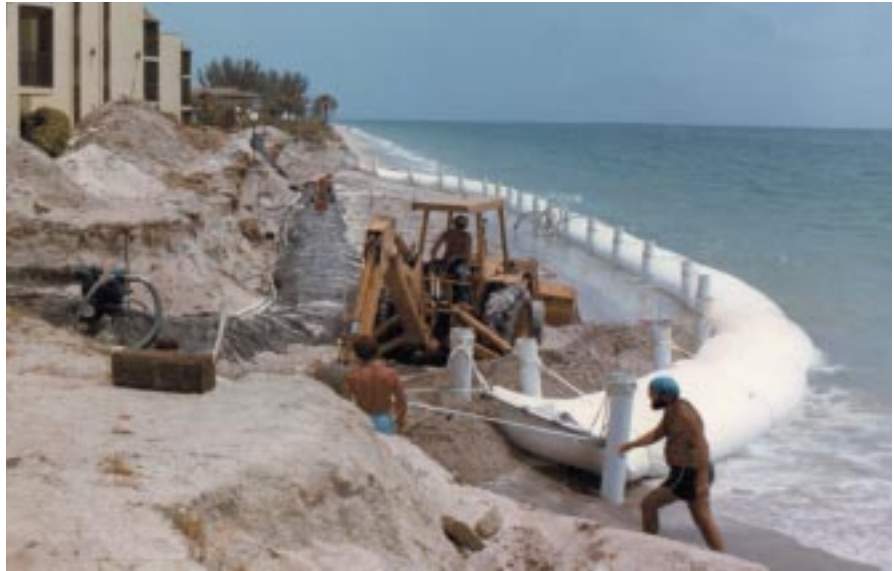
Photo 1: The first beach erosion-control solution, a round water-filled geotextile tube cofferdam, posed design challenges.
