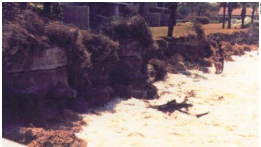
Photo 2: The eroded shoreline of the Longboat Key condominium before installation of the wedge-shaped geotextile-tube erosion-control structure.
