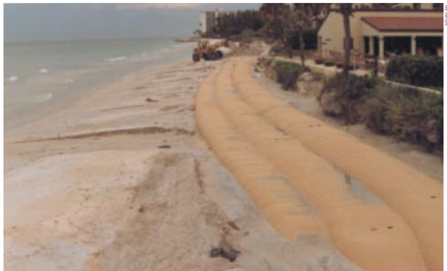
Photo 3: The progressively increasing tube heights of the wedge-shaped geotextile-tube structure, here shown installed in the beach of the Longboat Key condominium, deflect wave forces upward.
